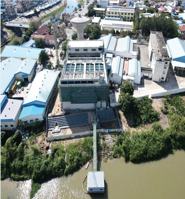
Install Equipment & Piping of Water Supply System In Ta Khmau - Cambodia Project
