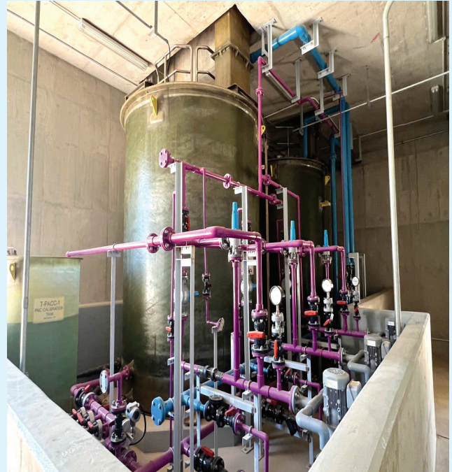
Install Tank & Piping of Water Supply System In Ta Khmau - Cambodia Project
