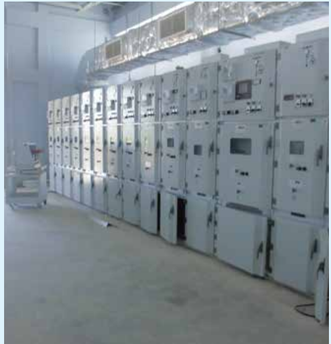
Medium Voltage Switchboard for Ton Hoa Sen Project
